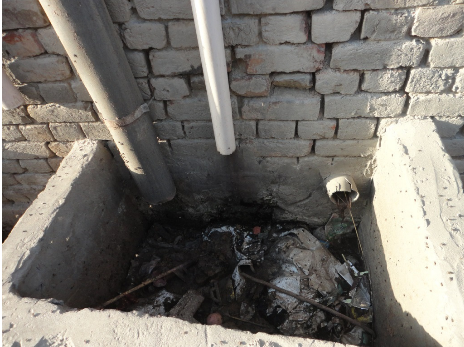
Figure 7: Waste Water Disposal in Farooqabad
