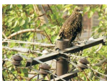
Fig. 12: Electrocutted Pariah kite on the electric pole
